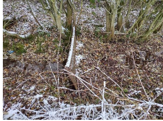
Figure 2.2 Grate crossing channel causing trapping of organic debris and backing up of water (looking from left bank to right at SP 52927 26132)
